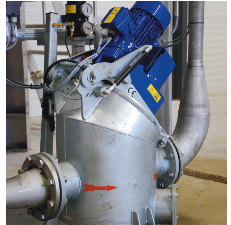
The mixed manure is pumped through a macerator, which ensures that larger particles such as teeth, pieces of wood and the like are grinded so that they do not log the system and cause unnecessary downtime.
