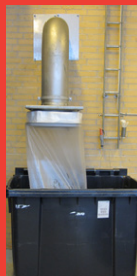
Discharge of compressed screen materials into Longofil bags which are well-suited as disposal bags for screen material. Continuous liner of plastic bags.
